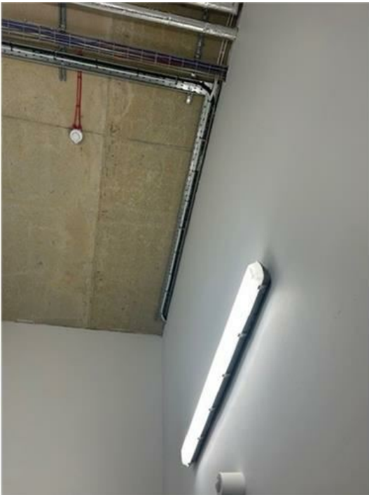
Hazel Bailey Holes in Bawtree wall.jpg
