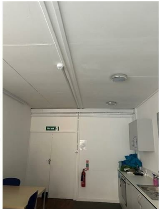
Hazel Dining tech room no Fire Blanket 2.jpg
