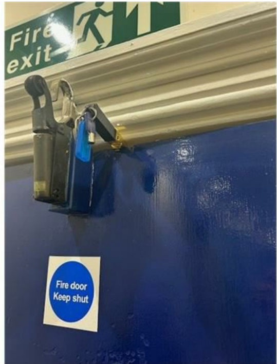
Hazel Main excessive door gap 2.jpg
