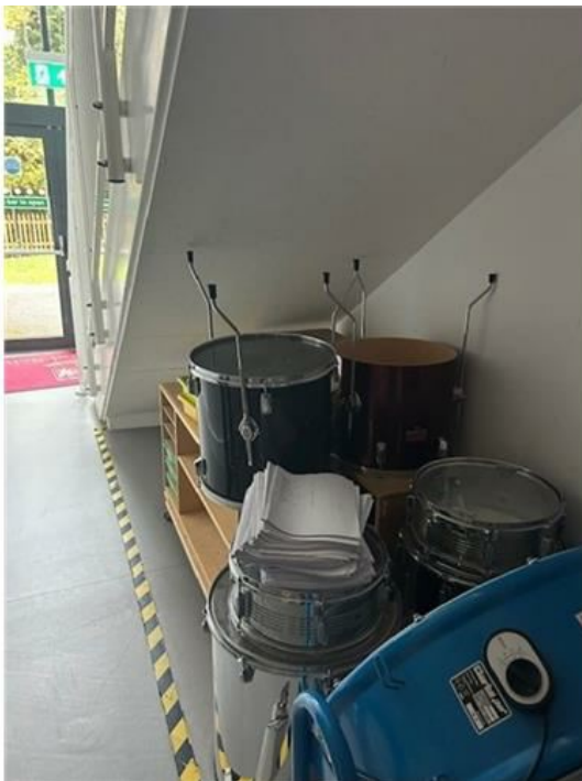
Hazel Bailey Combustibles in protected staircase.jpg
