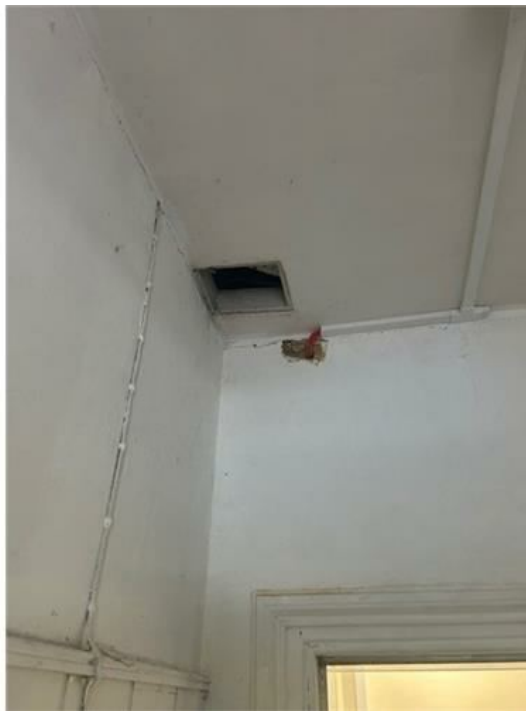
Hazel Main hole in laundry room ceiling.jpg
