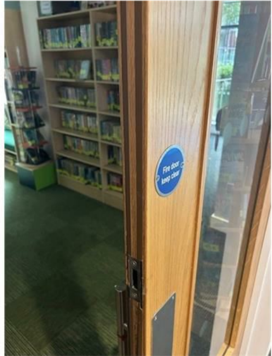
Hazel Bailey smoke seal missing - damaged Library 2.jpg
