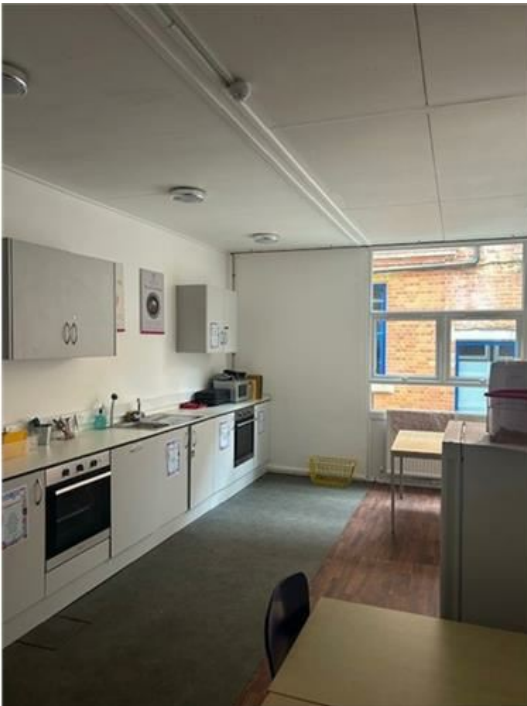
Hazel Dining tech room no Fire Blanket.jpg
