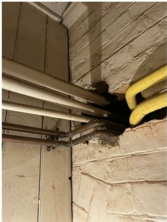
Hazel Main no Fire stopping 2.jpg
