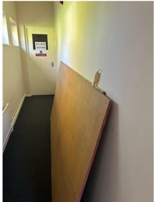
Hazel Meadow combustibles in protected hallway.jpg
