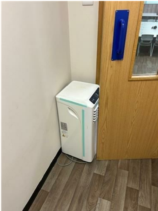
Hazel Elm FD blocked by Air Con blower.jpg
