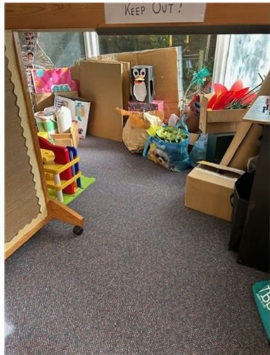
Hazel Forest Combustibles in Protected staircase 2.jpg
