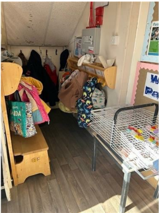
Hazel Meadow combustibles in protected staircase.jpg
