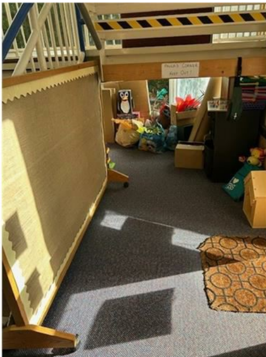
Hazel Forest Combustibles in Protected staircase.jpg
